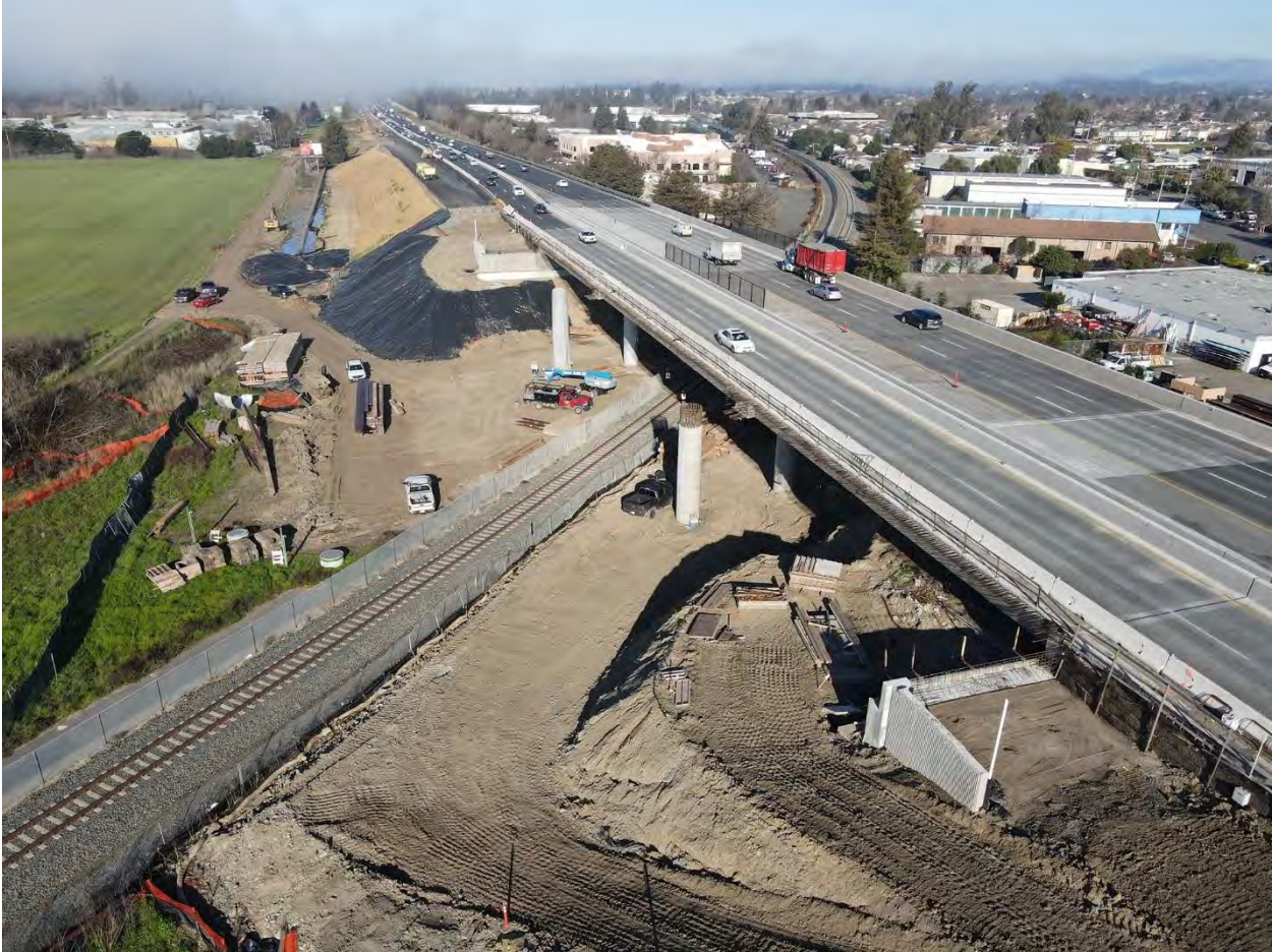
Replacement of the North Petaluma Overhead, Highway 101 over SMART Under construction in 2022
