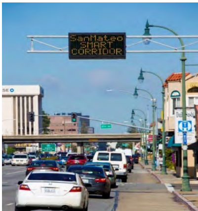
Pictured: Intelligent Transportation System (ITS) equipment along the San Mateo County Corridor.
