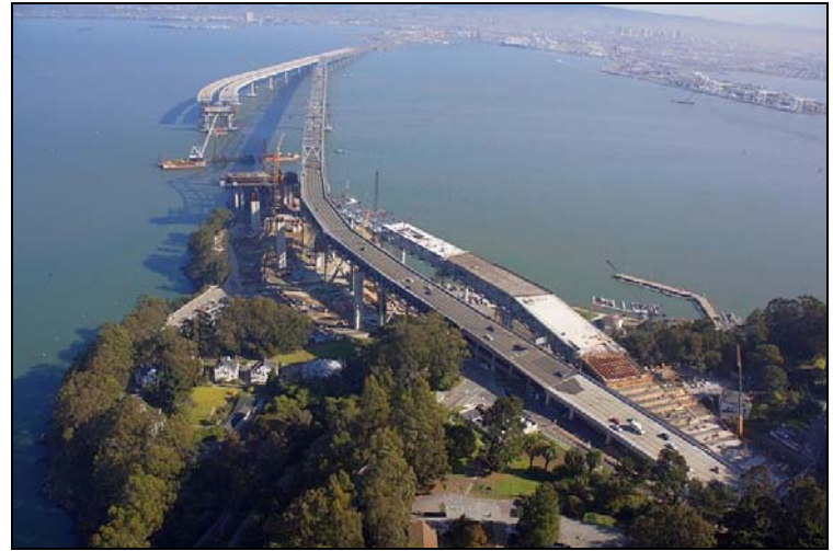
Aerial View of the East Span of the SFOBB from Yerba Buena Island
