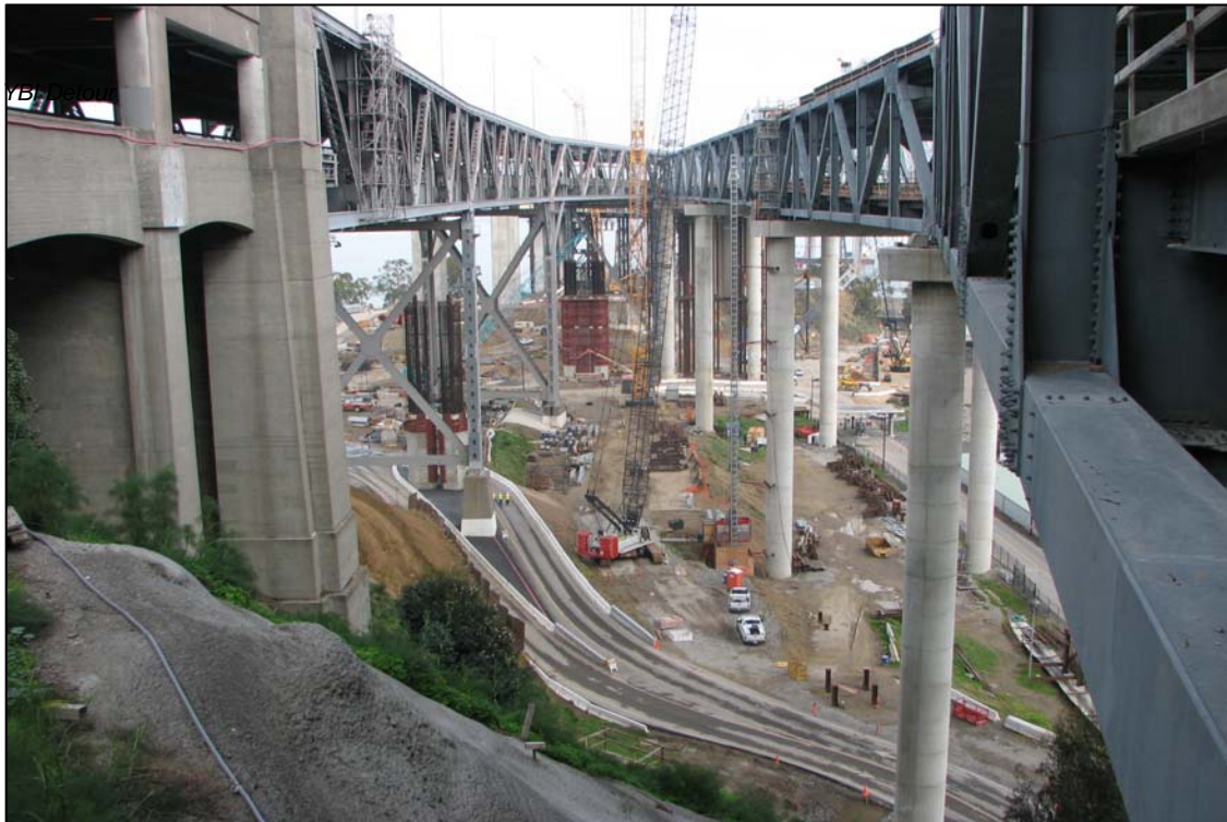
Yerba Buena Island Transition Structures (YBITS) on the Left and Yerba Buena Island Detour (YBID) on the Right.
