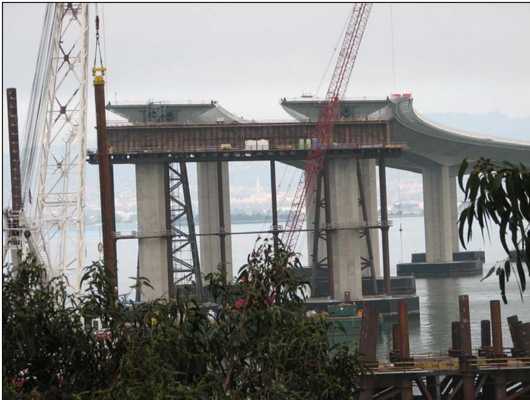
E2 Support Structure
