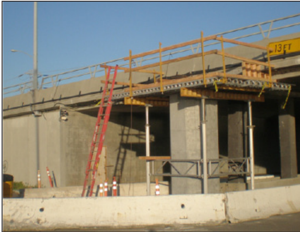
Falsework for Bent Cap Extension within Median of Frontage Road at the West End of the Project
