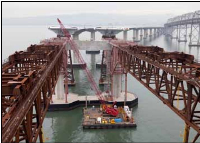
Temporary Support Structures with E2 Cap Beam and Completed Skyway in background
