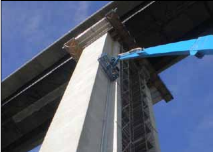
Antioch Bridge - Installation of Seismic Monitoring Conduit along Height of Column Bent at Pier 22
