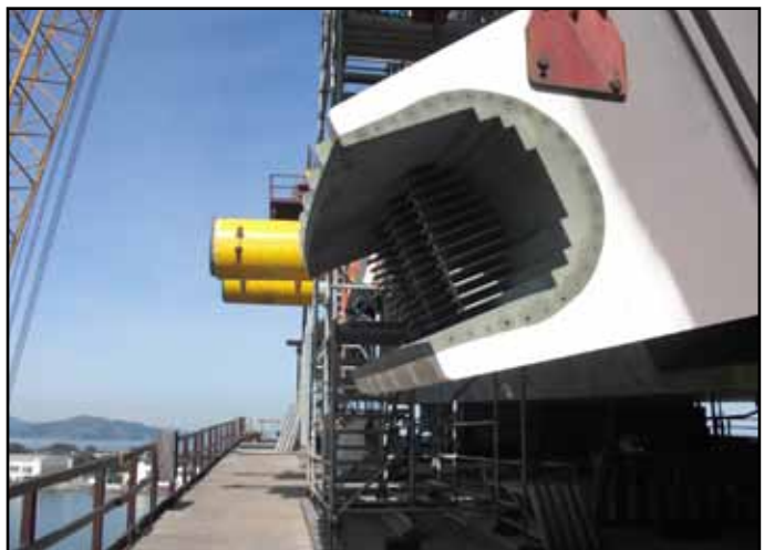
Recently Erected Jacking Saddle and Hinge K Pipe Beams at Hinge K on Yerba Buena Island
