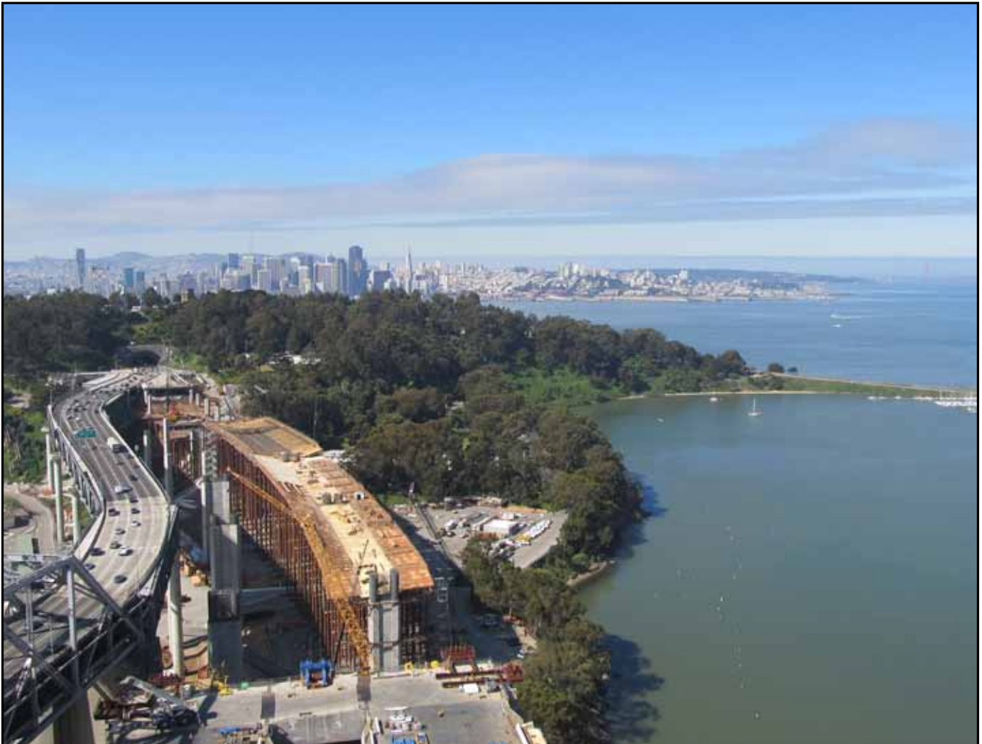
View from the SAS Tower Overlooking YBITS #1 Westbound Falsework and Formwork Progress on Right and Existing Bridge on Left
