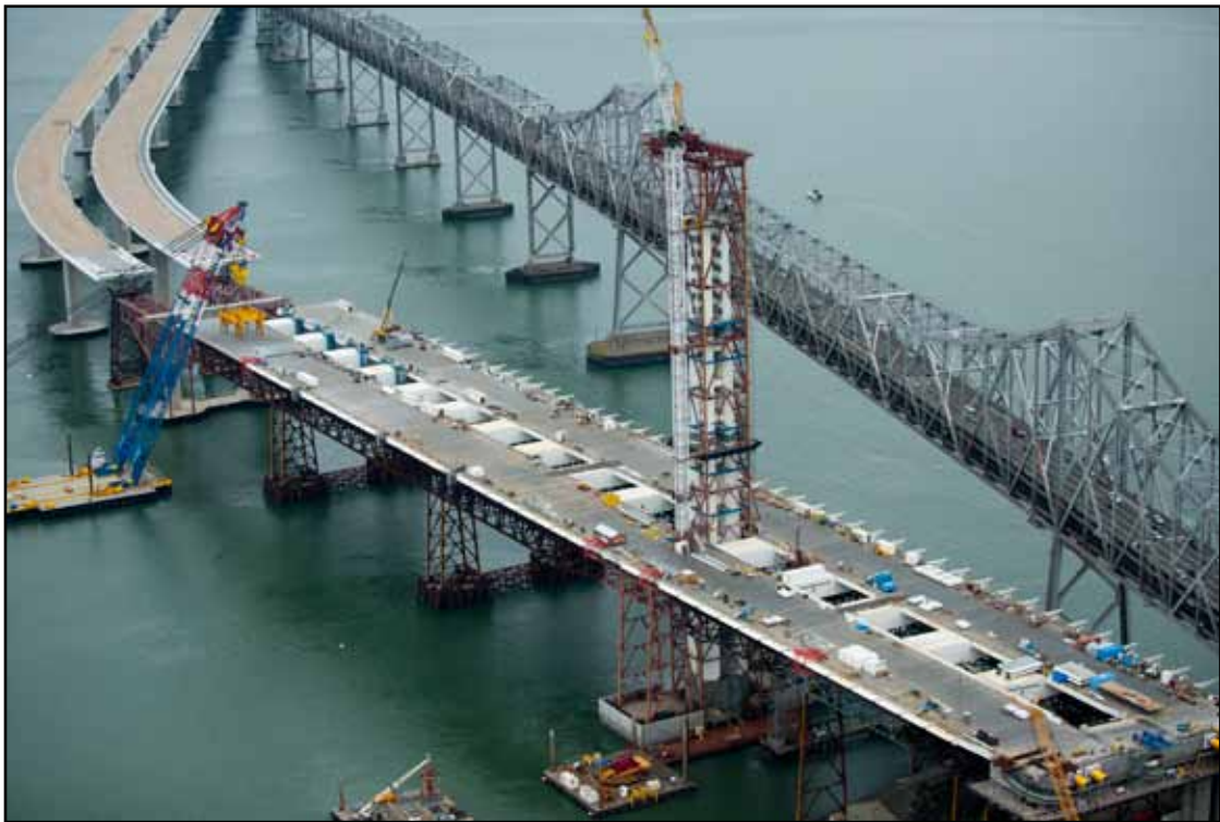
Aerial View of Roadway Box 11 E Being Installed and the First Leg of the Fourth Tower Lift Erected
