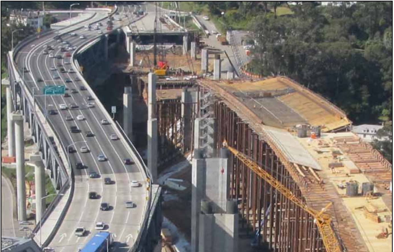
Yerba Buena Island Transition Structures #1 Falsework and Form Work in Progress on right and Yerba Buena Island Detour on the left Looking West
