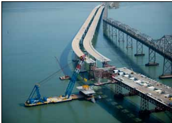
Aerial View of Roadway Box 11 Westbound Being Lifted into Place by the Shear-Leg Barge Crane
