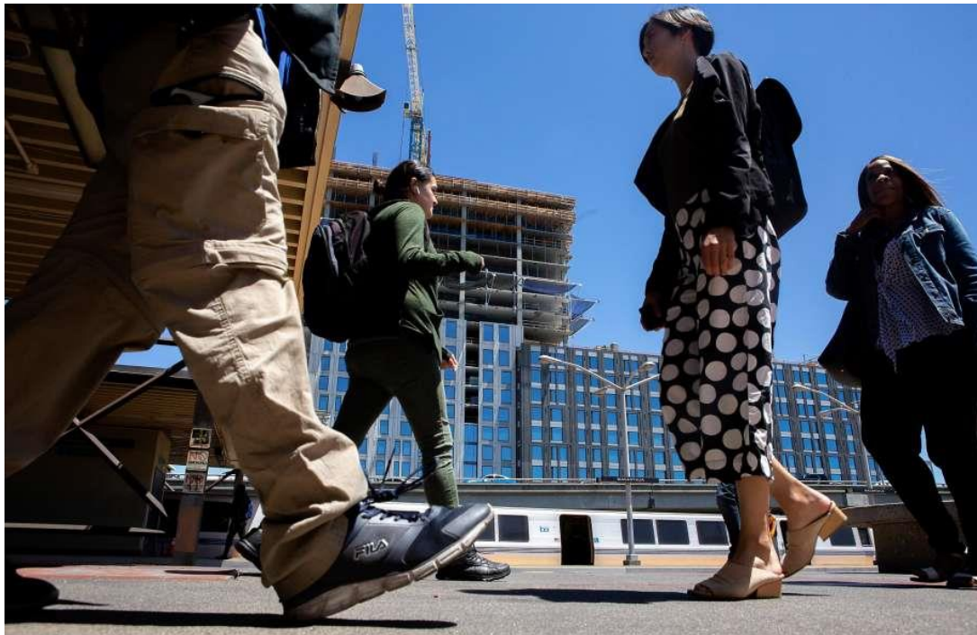
The MacArthur Transit Village under construction near the BART station platform. Future transit villages can further integrate mobility hub design and amenity features using overlay zoning.
