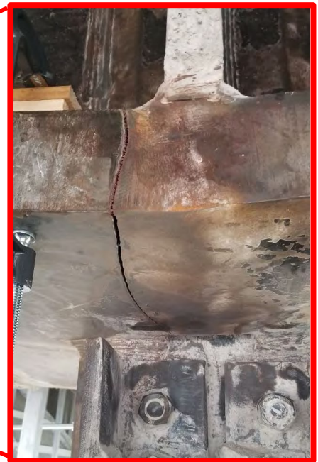
3. Fracture through bottom flange
