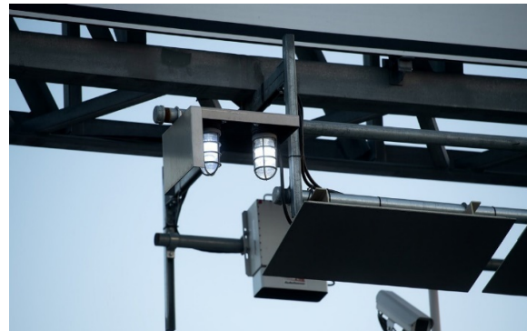
Figure 3: Close-up of Toll System Equipment (photo courtesy of Noah Berger)
