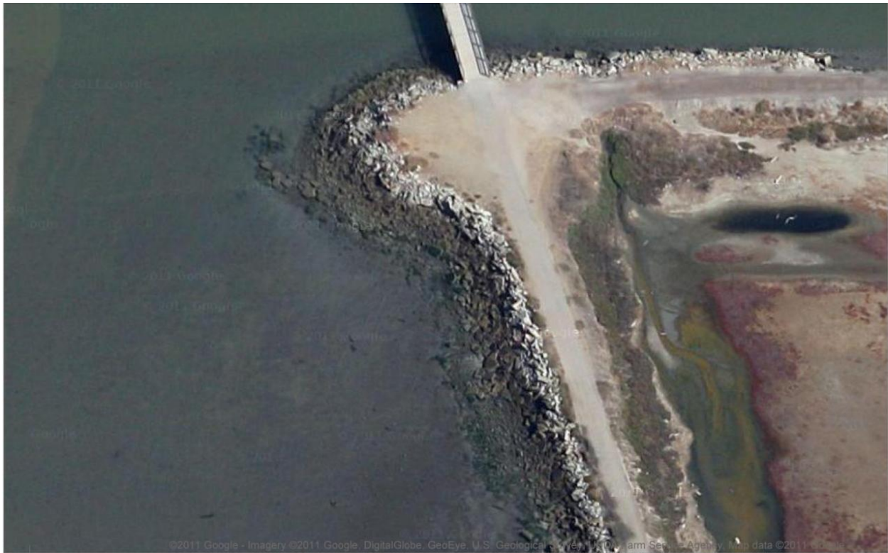
Figure 2.10 Nonengineered Berm with Riprap Protection, Hayward; Roadway Berm Is Berm Crest
