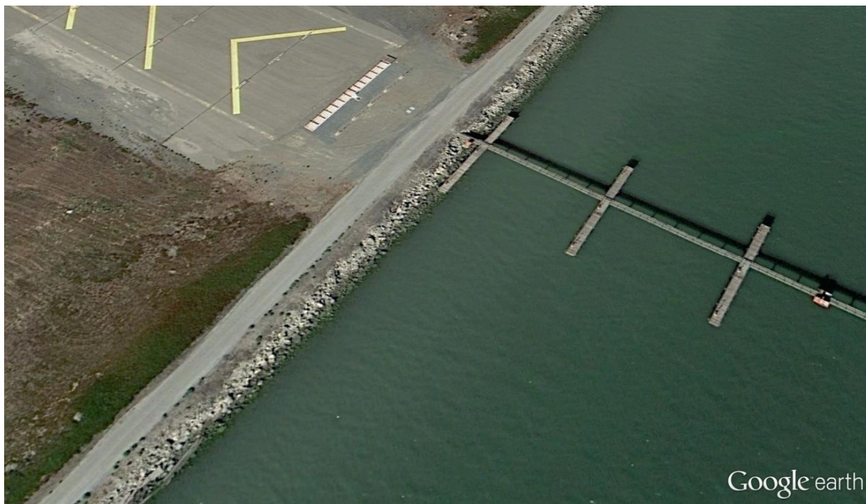
Figure 2.4 Engineered Levee with Revetment: Oakland International Airport, Oakland; Roadway Is Levee Crest
