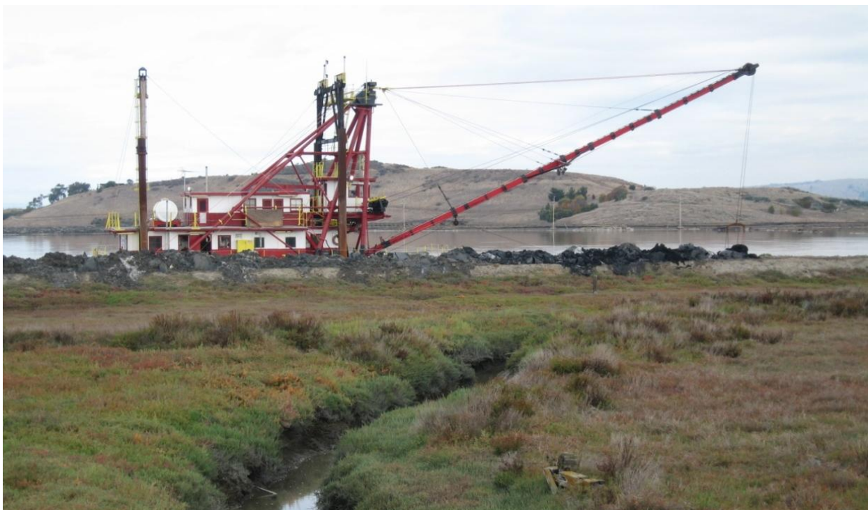
Figure 2.12 Maintenance of a Nonengineered Berm in Eden Landing by the Mallard, Hayward
