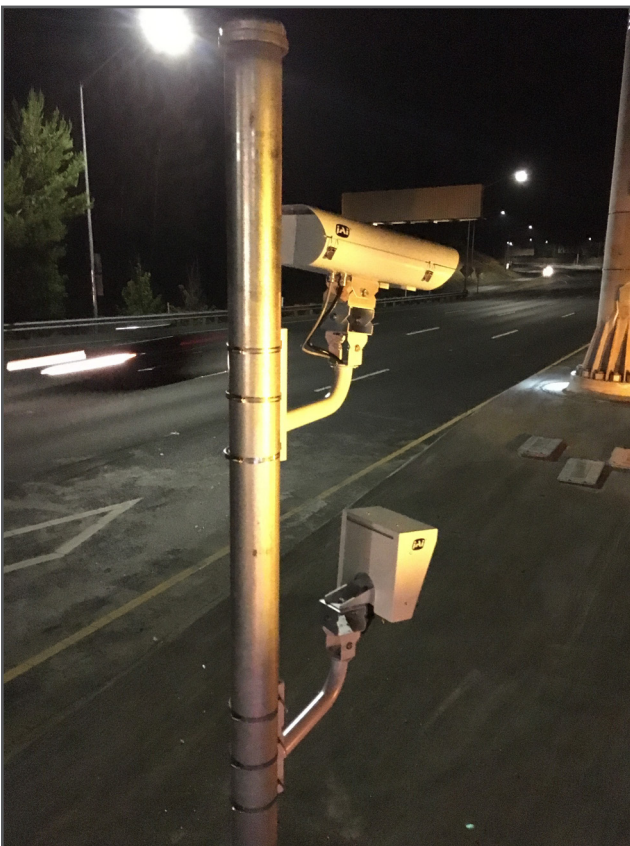
Violation camera for the toll system.
