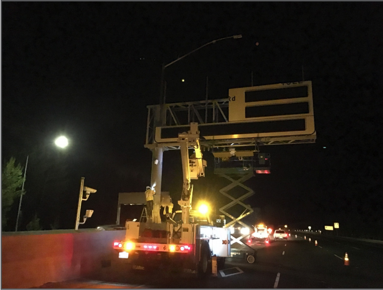
Construction crews work on connecting toll system components to Variable Message Sign on I-680.
