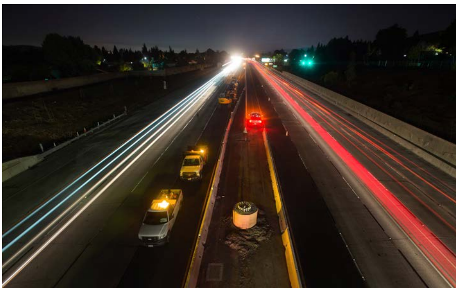
A completed CIDH (Cast-In-Drill-Hole) structural foundation for an express lane sign placed in the future reconstructed median barrier of I-680.
