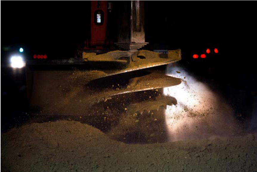
Drill attachment pushes through the earth to pre-drill shafts for the express lane sign foundations.
