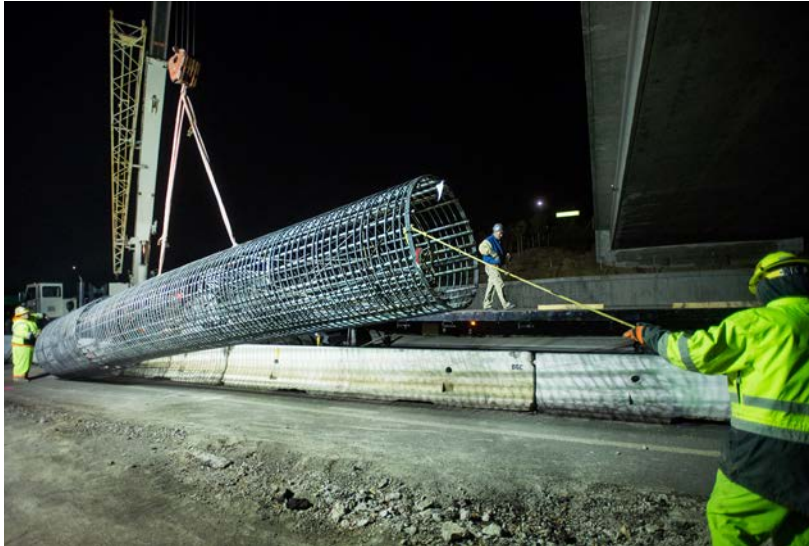
A crane picks up a pre-fabricated rebar cage to place in the pre-drilled shaft to reinforce the concrete for the express lane sign foundations.
