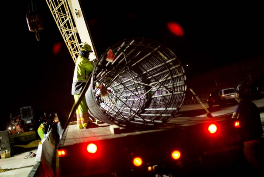
Construction crews unload a pre-fabricated metal rebar cage. This cage reinforces the foundations once concrete is poured.
