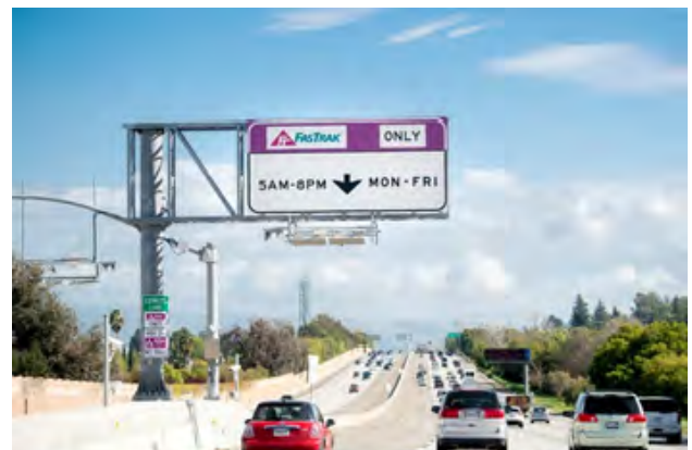
Overhead hours of operation sign and toll system equipment on the I-680 Express Lanes
