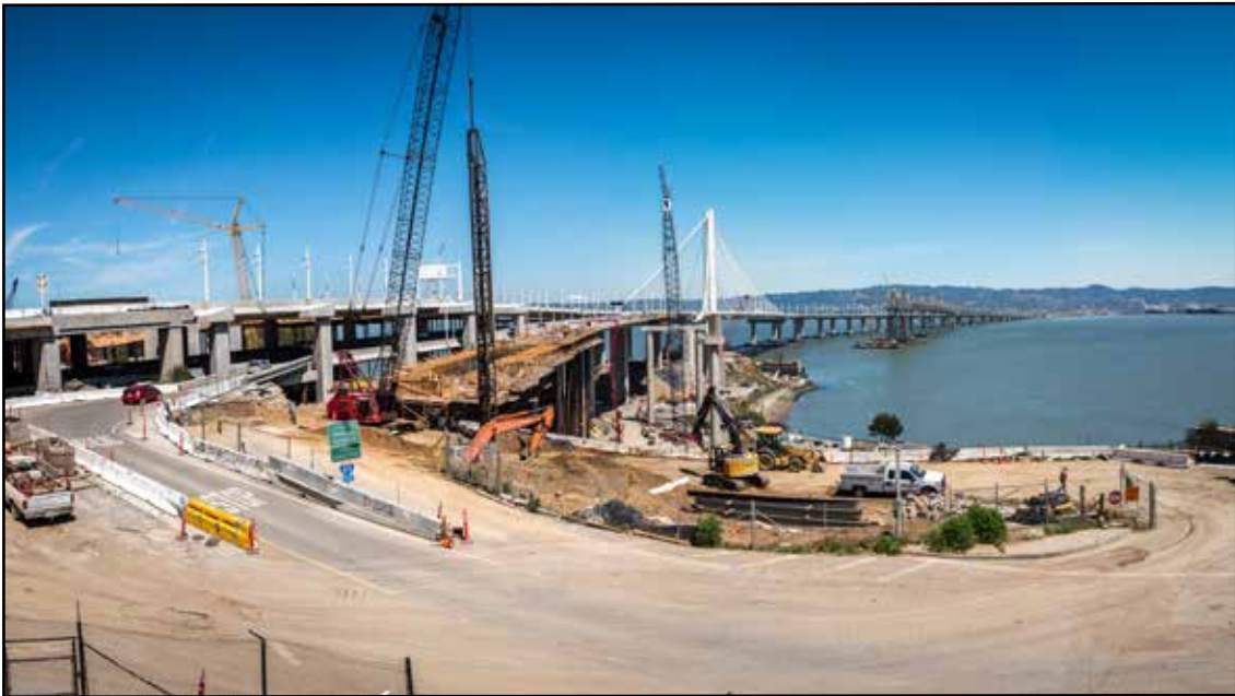
Eastern Span of the San Francisco-Oakland Bay Bridge Bicycle/Pedestrian Path and Ramp Construction in Progress
