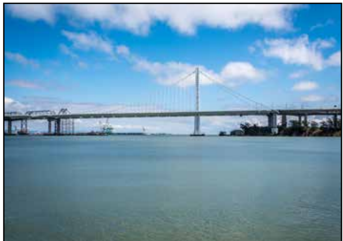
View of the New Bridge as Old Bridge Continues to be Dismantled
