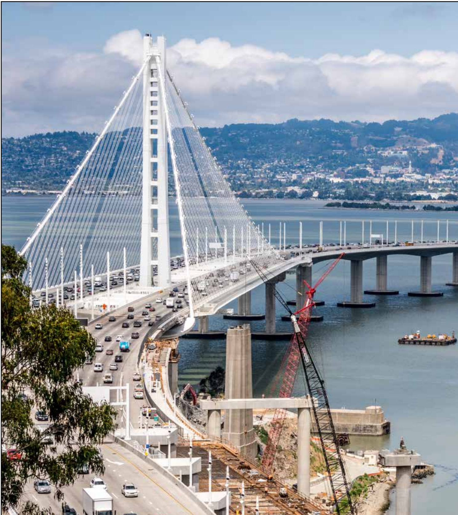
Yerba Buena Island Transition Structures Demolition Progress on right with the New Self-Anchored Suspension Span of the San Francisco-Oakland Bay Bridge on Left Looking east toward Oakland
